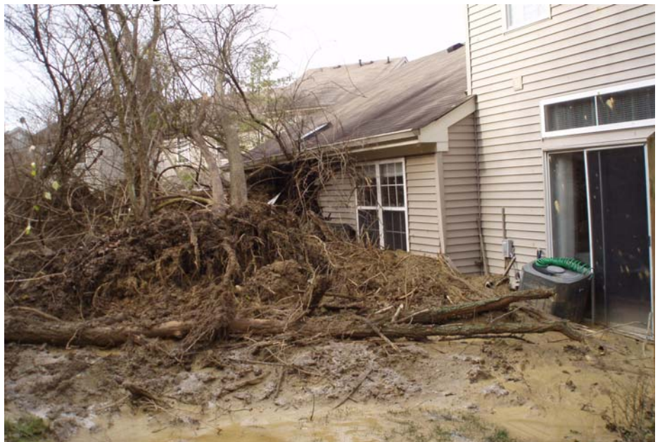
Rotational landslide damages Clifton home
